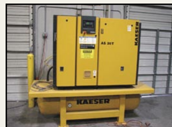
KAESER AIR COMPRESSOR
